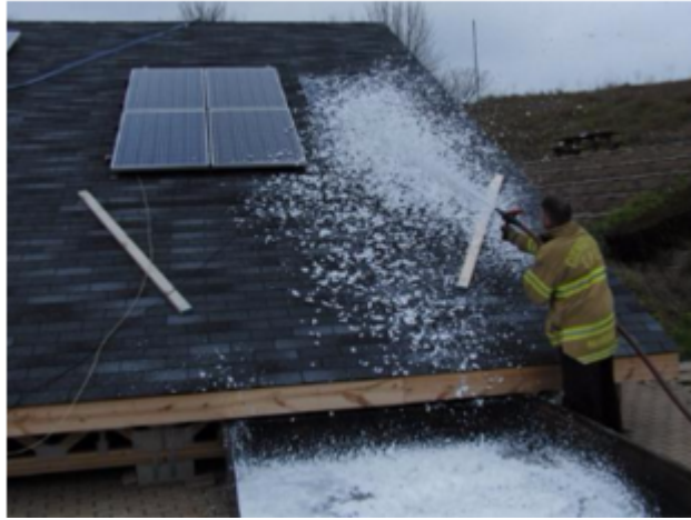
Figure 17: Firefighters Applying Foam to Solar PV Panels (Backstrom & Dini, 2011)
