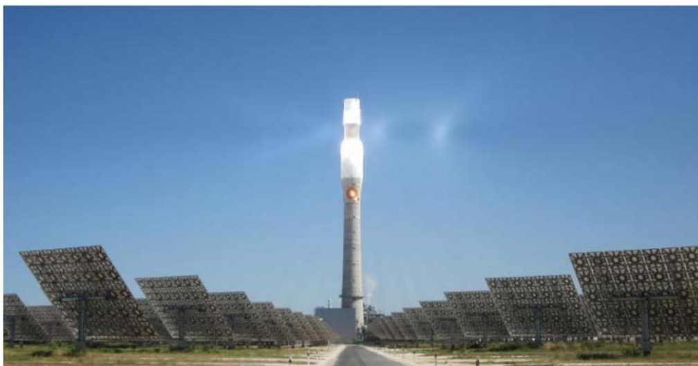
Figure 5: Concentrating Solar Thermal power station.
