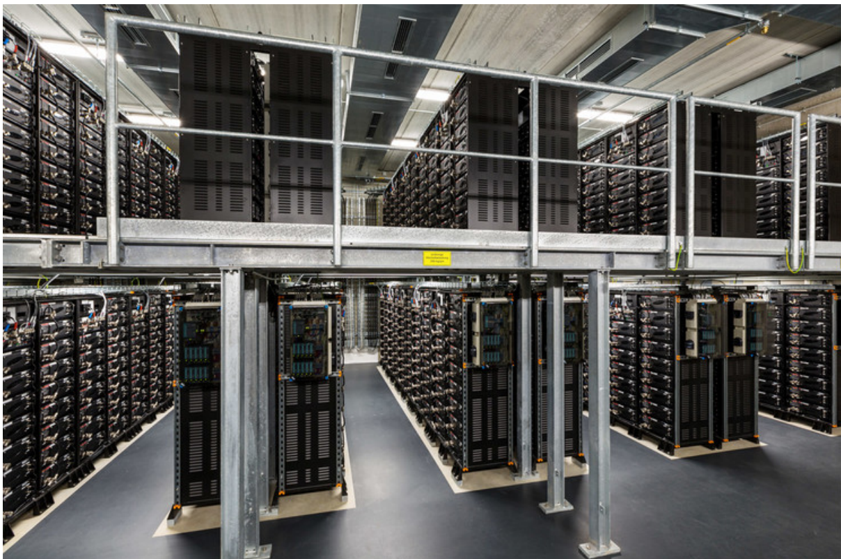
Figure 6: Battery plant at Schwerin, Germany.
