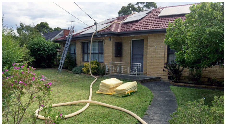
↑ The granulated Rockwool is pumped into wall cavities from the top, or through holes in the wall which are later filled.
