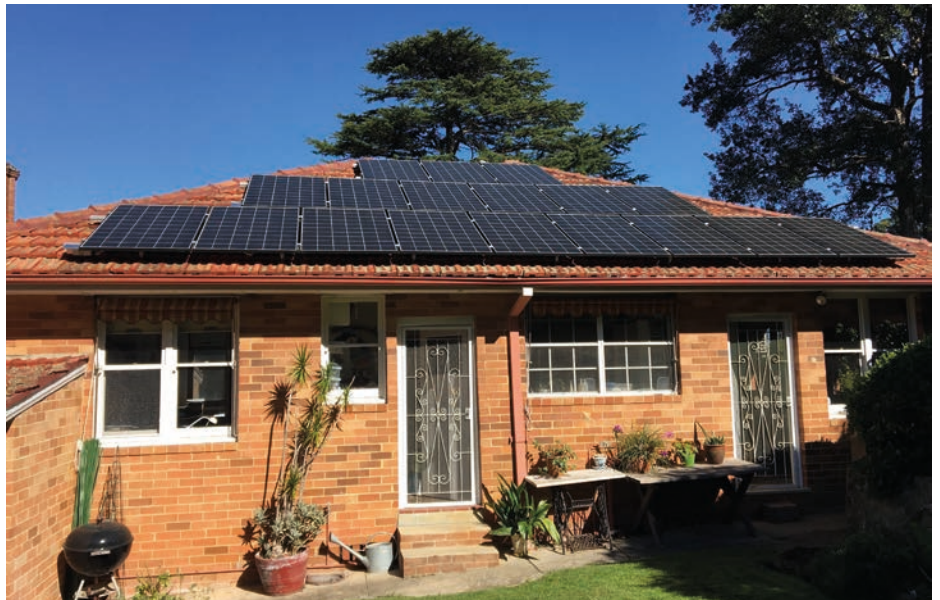
The view from the backyard is quite impressive, as the north-east array has filled almost all available roof space.
