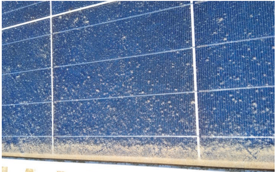
Dust can build up on solar panels to the point where power output can be noticeably affected. These panels, in a rural area, hadn't been cleaned in almost five years, with energy output down around 6%.
