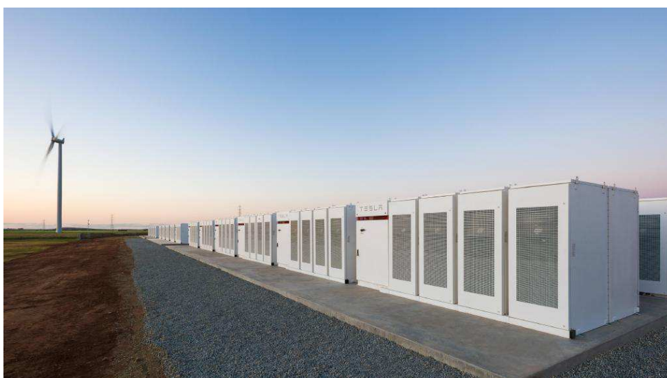
Figure 6: Jamestown Tesla battery
