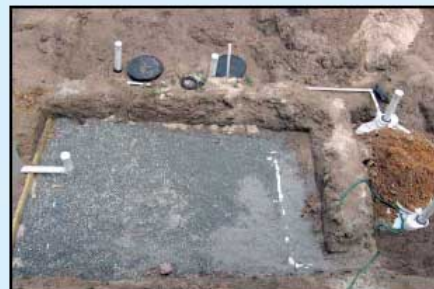
7. The sand filter system is complete and ready to be covered by lawn.
