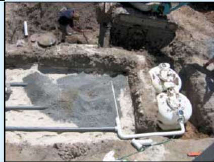
6. Pipes distribute greywater over the total area.
