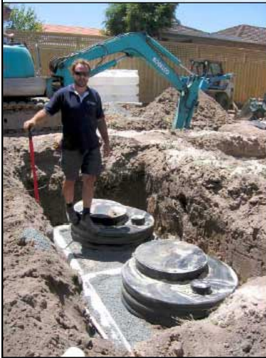
4. Two pump wells are required. One captures the greywater and pumps it to the settling tank (top). The second well captures treated greywater from the garden, ready to be sent to the irrigation system.
